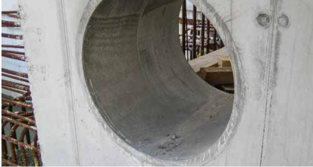
FZR400/300 Installation location sewage treatment plant
