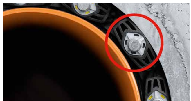
GKD with one segment not tightened - installation error immediately detected.
