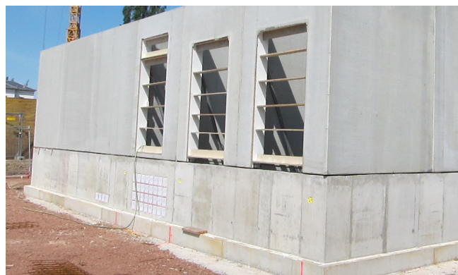
After concreting the basement on-site, the service building was erected using prefabricated concrete walls.
