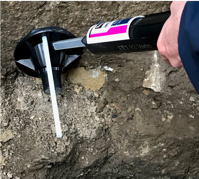
The entry is properly sealed to the outside wall using two-component expansion resin injected into a 30 mm opening in the building.
